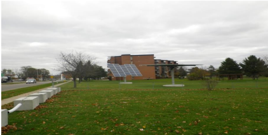
Ground Mounted Solar Panels at Trillium Way, Paris
